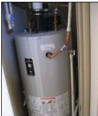
23. View of typical water heater in the water heater closet.
