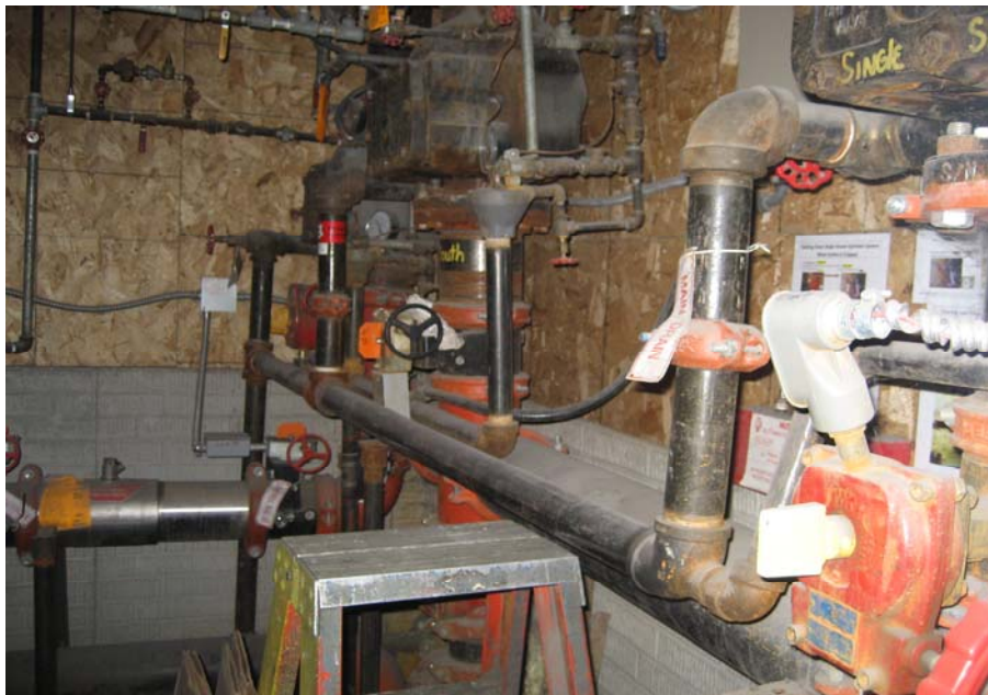
Photograph No. 10 Fire backflow system
