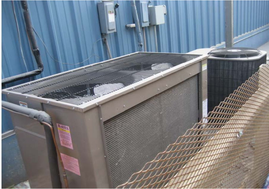
Photograph No. 15 Typical HVAC units
