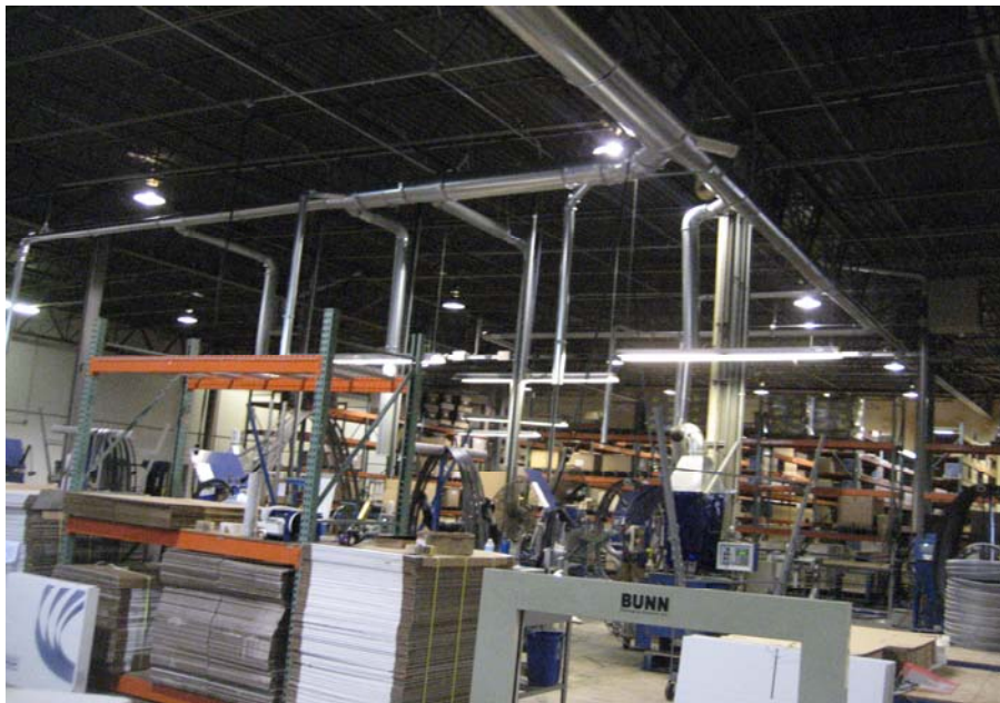
Photograph No. 22 Clean Air ventilation system at the Property.
