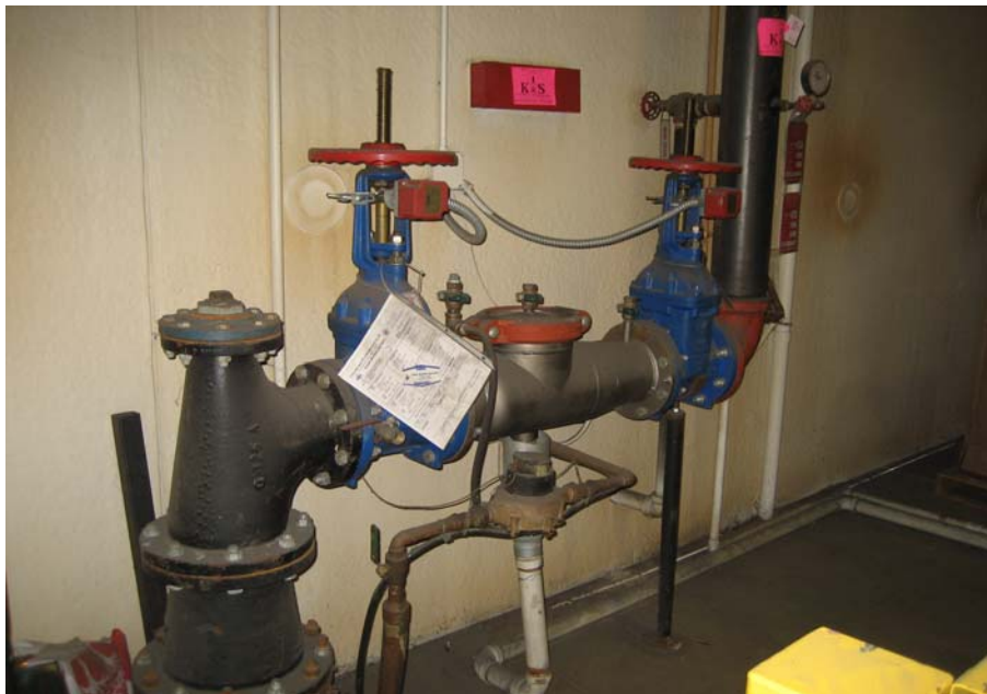
Photograph No. 10 Fire backflow system
