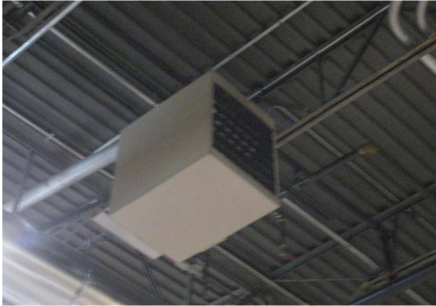
Photograph No. 27 Typical HVAC system at the Property.
