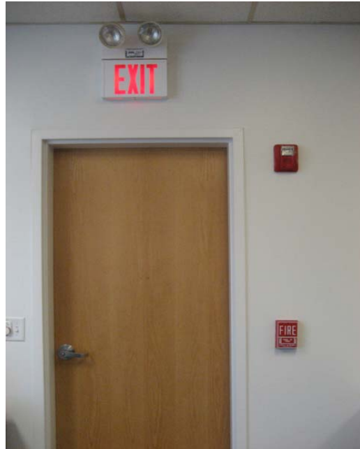
Photograph No. 11 Typical fire alarm and emergency exit.
