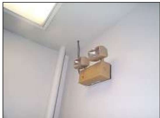
18. Emergency lights throughout building
