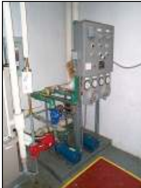
25. Pumps for domestic water system
