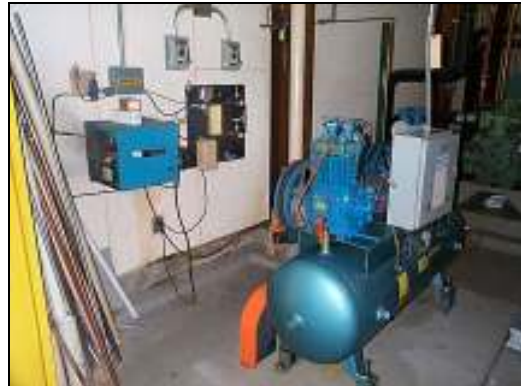
32. Compressor system for pneumatic HVAC controls
