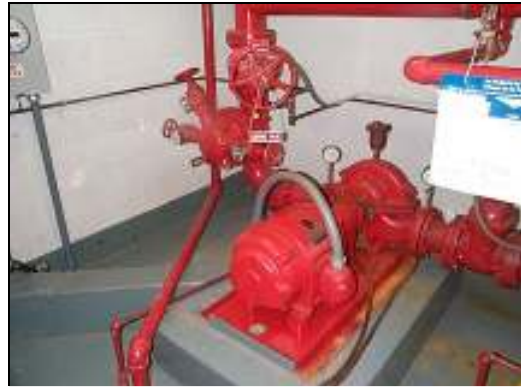
22. Fire sprinkler pump
