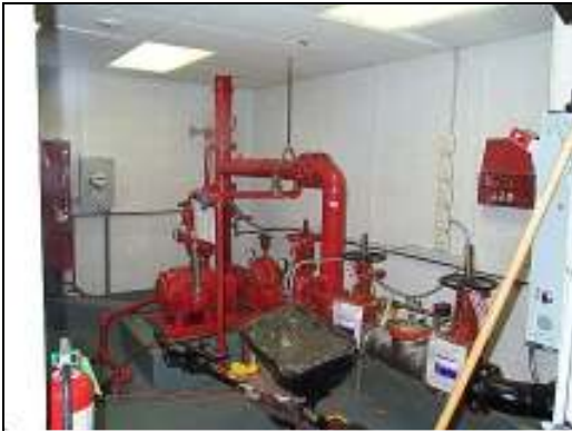
19. Fire sprinkler riser and equipment room
