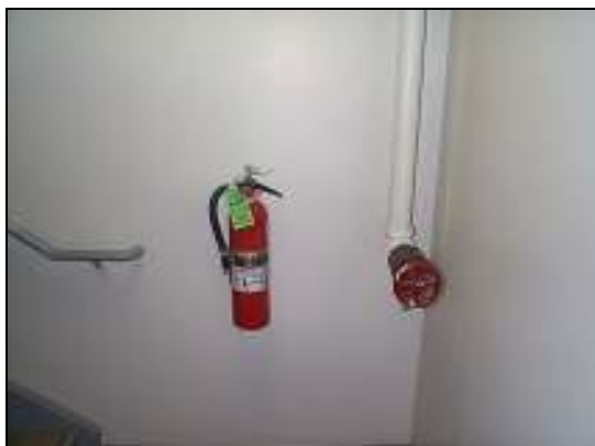
17. Life safety equipment in stairwells
