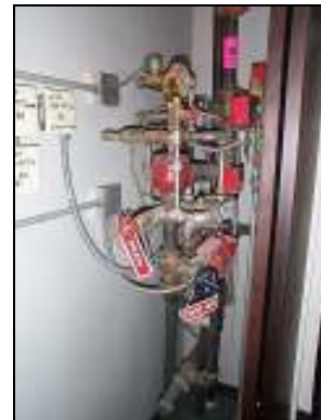
28. Dry sprinkler system for tenant computer room located on 4 th floor
