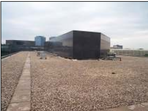
33. Roof – mechanical penthouse
