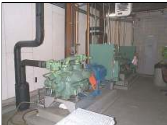
29. HVAC penthouse with Carrier Compressors
