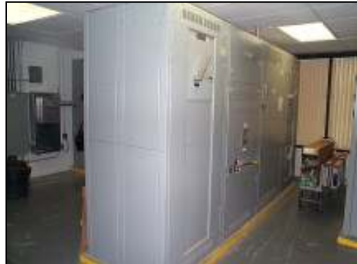
26. Main electrical room
