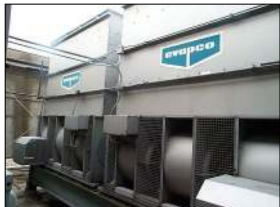
30. Two 150-ton cooling towers
