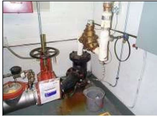
20. One main incoming water line
