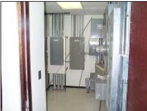
27. Typical electrical meter room and tenant breakers on each floor
