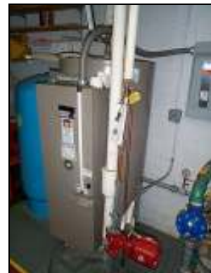
24. Electric water heater with new pump
