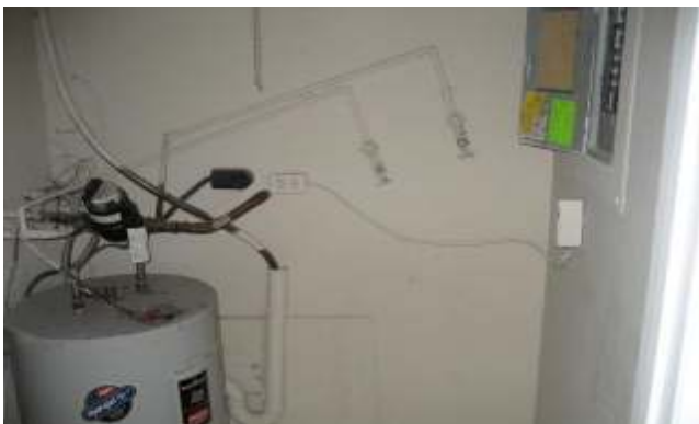
23. View of typical laundry connections in the water heater closet.
