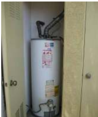
23. View of typical water heater in the water heater closet.
