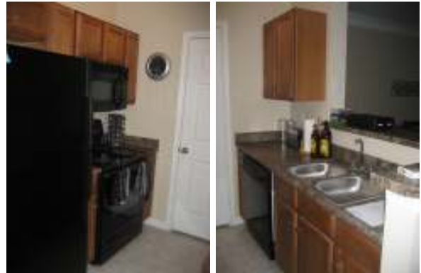
14. MICROWAVE VENT HOODS AND ELECTRIC RANGES IN KITCHENS
