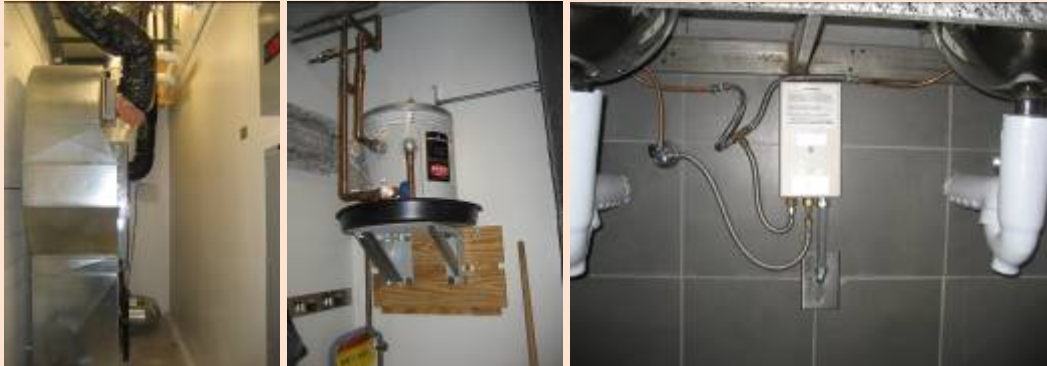
HVAC System and Water Heaters at the Property
